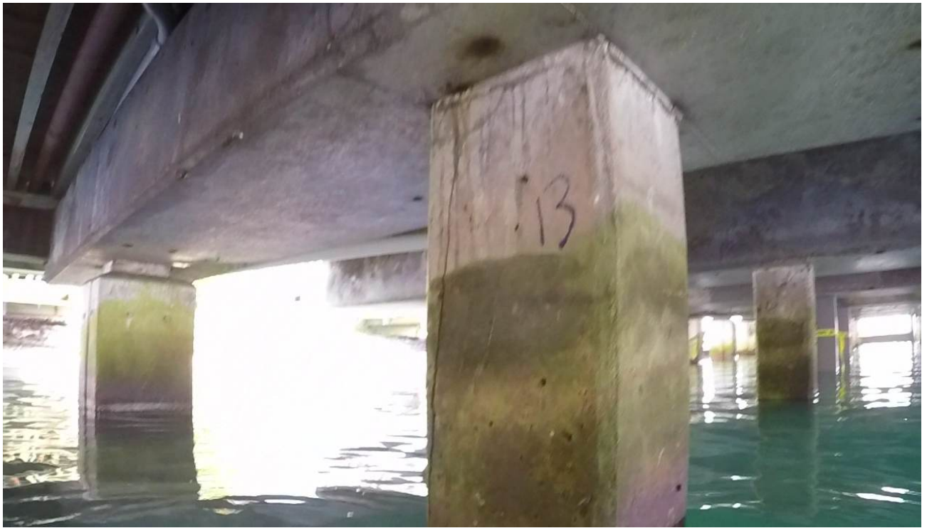
Concrete Dock Piles Sign of Deterioration
